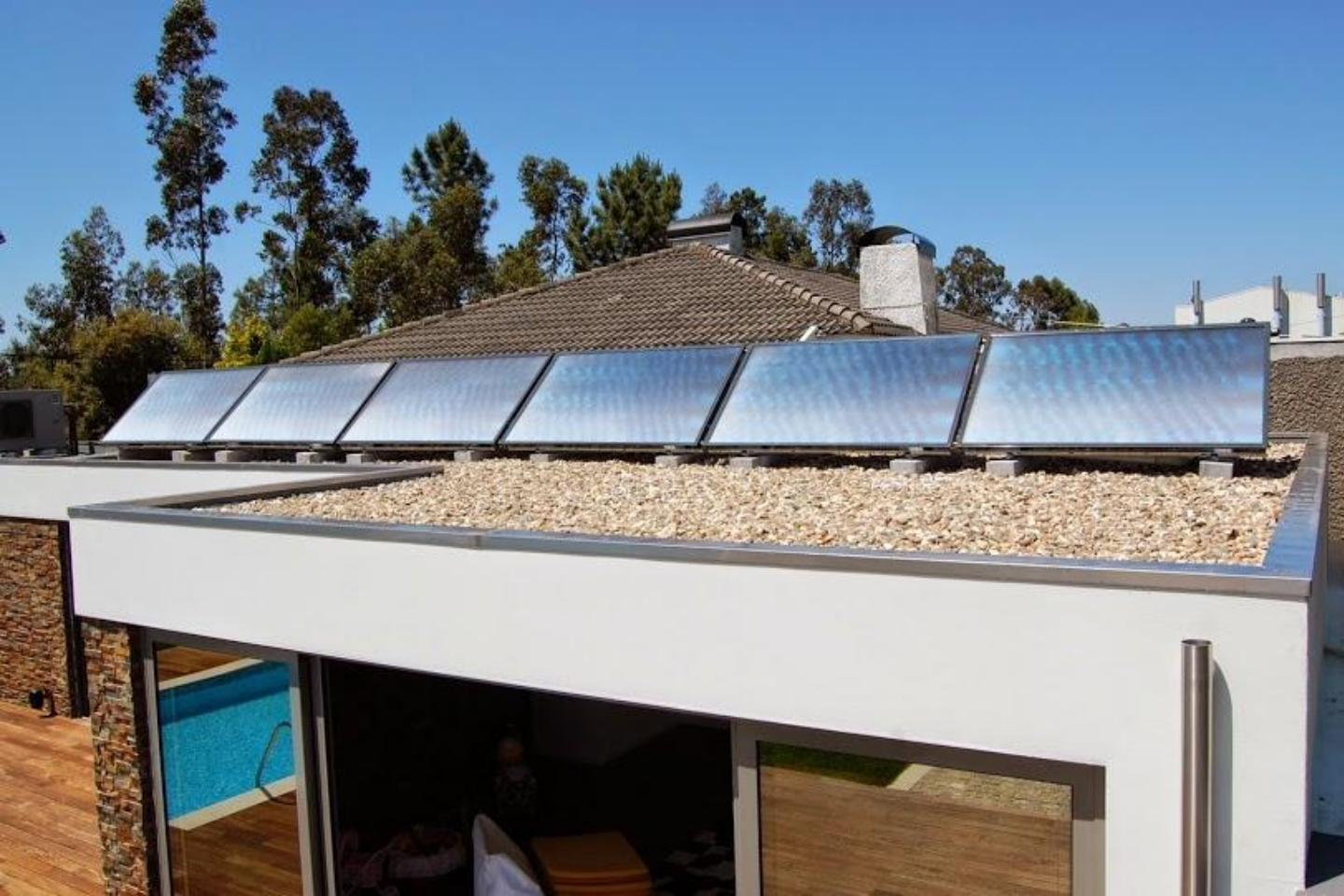
Solar Water Heaters
